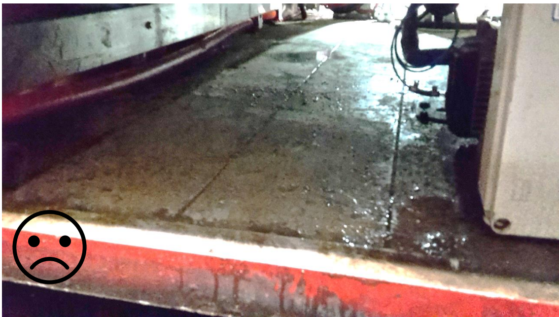
Figur 19. Magasin-/teknikrum med skidt/gødning – AFVIST / Storage compartment/technical control compartment with dirt/manure – REJECTED.
