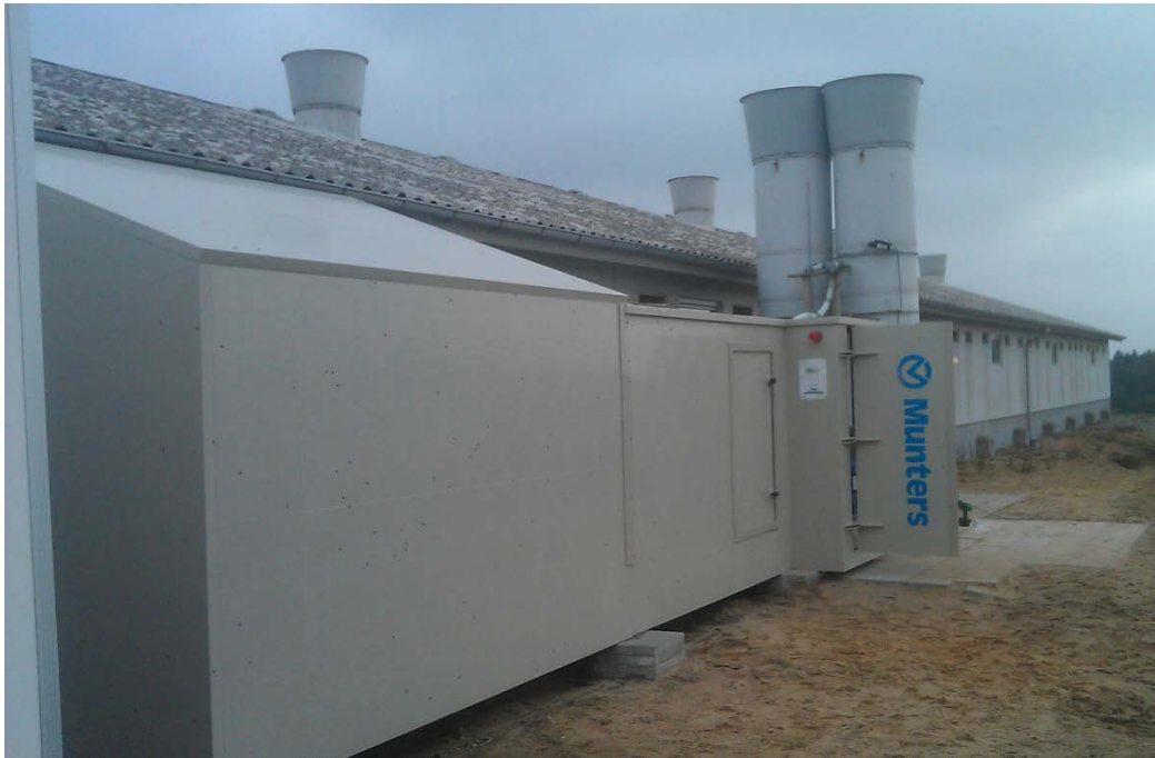
Figure 1. MAC 2.0, the air cleaner with acid from Munters A/S installed in a finisher unit.
