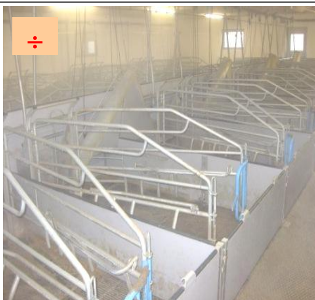
Farrowing facility poorly cleaned and still moist, and therefore not ready for sows
