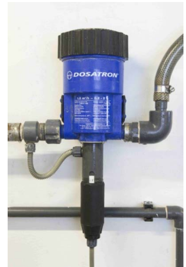
Use a medicator is for cleaning the water system
