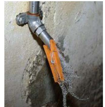
Activate all valves during disinfection
